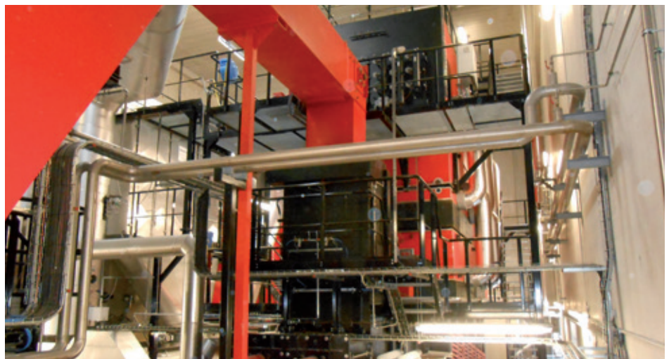
PDV biomass boiler
